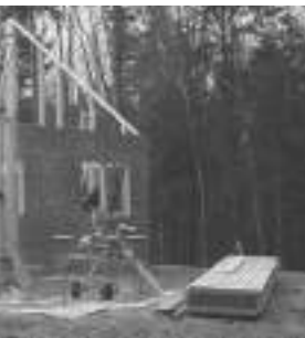
Har and crew working on the access road and around the hut.
